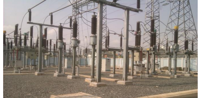
( Vietnam Power Company – Binh Tri Dong High Voltage Power Station)
